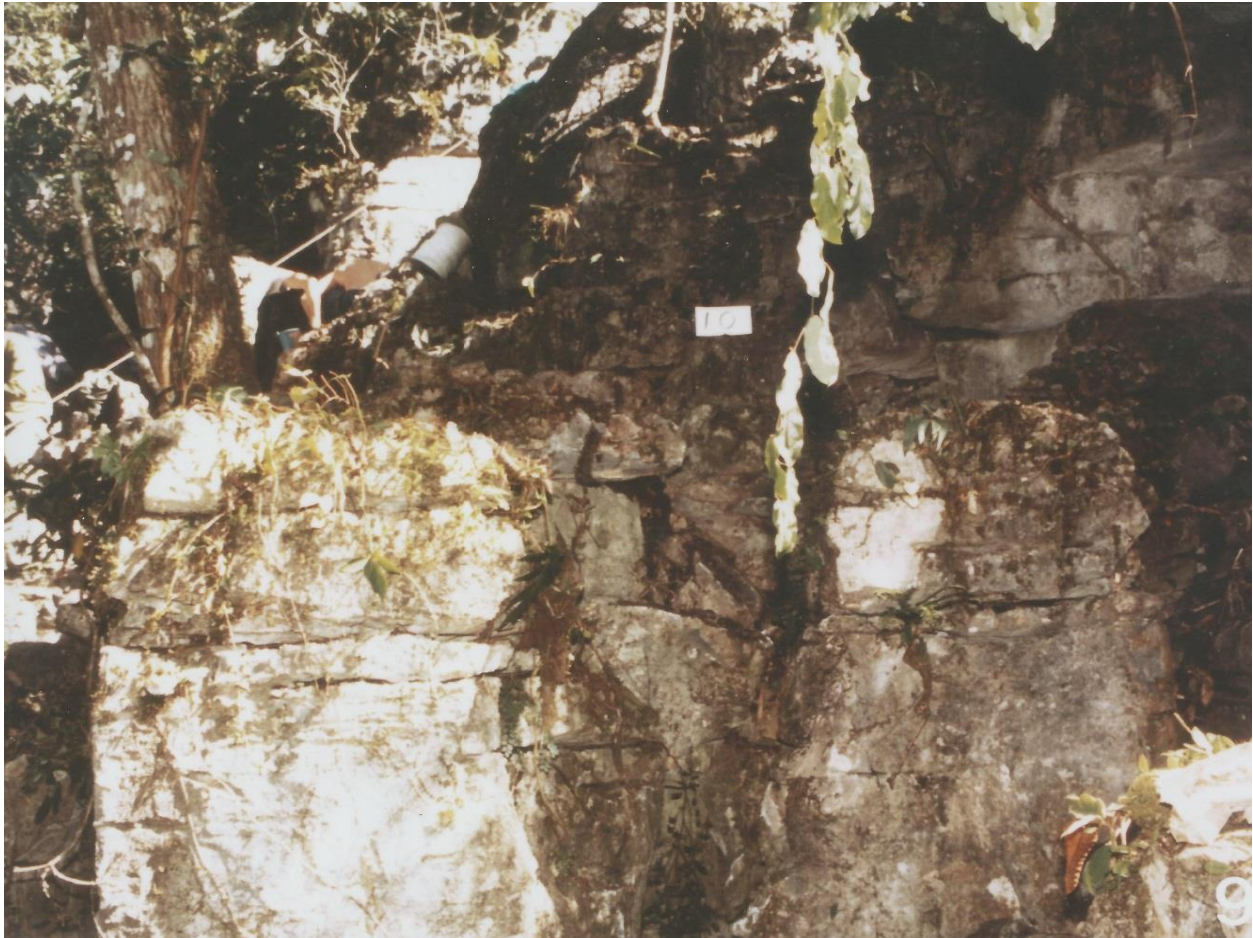
Rectangle marks the nose impact point. Note the stretched safety line on upper right.
